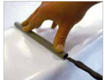
Install an electrical conduit through which the cable can pass under the coping (so the motor can be replaced in the future if necessary).
