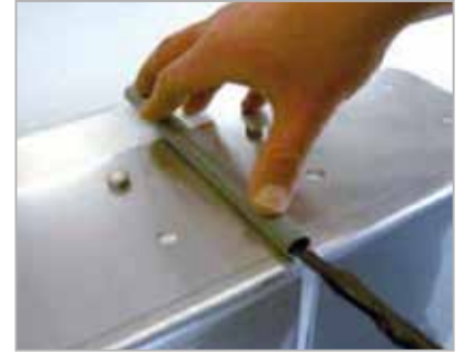
Install an electrical conduit through which the cable can pass under the edge tile (so the motor can be replaced in the future if necessary).
